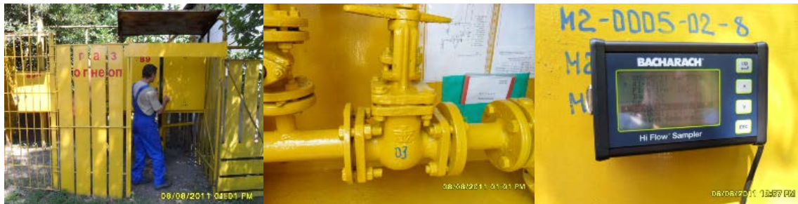
Figure 4 Cabinet Type Gas Regulation Point
