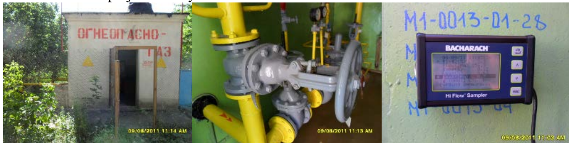
Figure 3 High Pressure Gas Regulation Point
